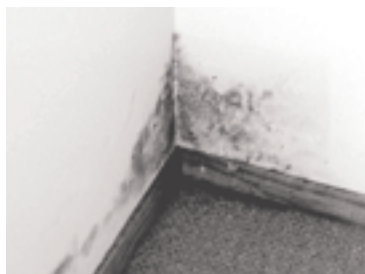
Condensation has led to mould problems on the drywall.
