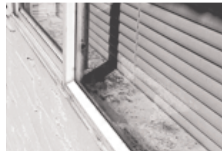
Evidence of problems resulting from condensation can be seen on the interior window sill.
